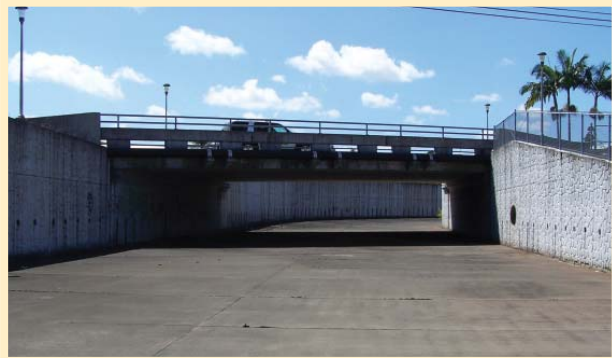
The flood channel in Kawaiilani Street Bridge was realigned and designed to hold more water.
